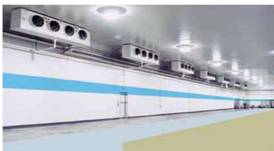
Figure 89: Multiple evaporators cool a large Cold Storage facility
