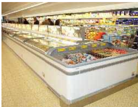
Figure 62: Self-contained high efficiency horizontal 'coffin' style freezer operating on natural refrigerants
