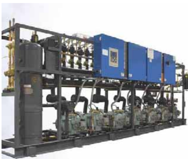
Figure 63: Typical parallel compressor rack
