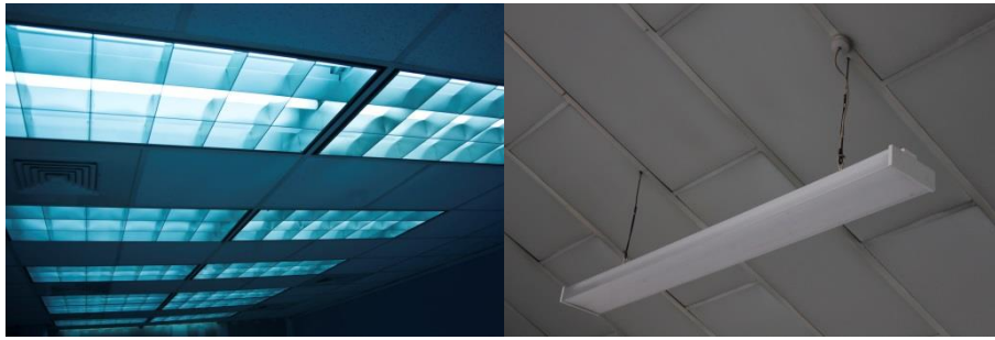
Figure 28: Recessed troffers with louvres to direct light output (left) and a pendant batten with diffuser (right)
